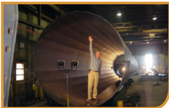
Hager City’s new long tandem press bends flat steel plates into 12- and 16-sided polygonal tubes, a critical part of the process for fabricating power transmission poles. Pictured is Bob Schultz, retired T&B Steel Structures vice president sales and marketing.
