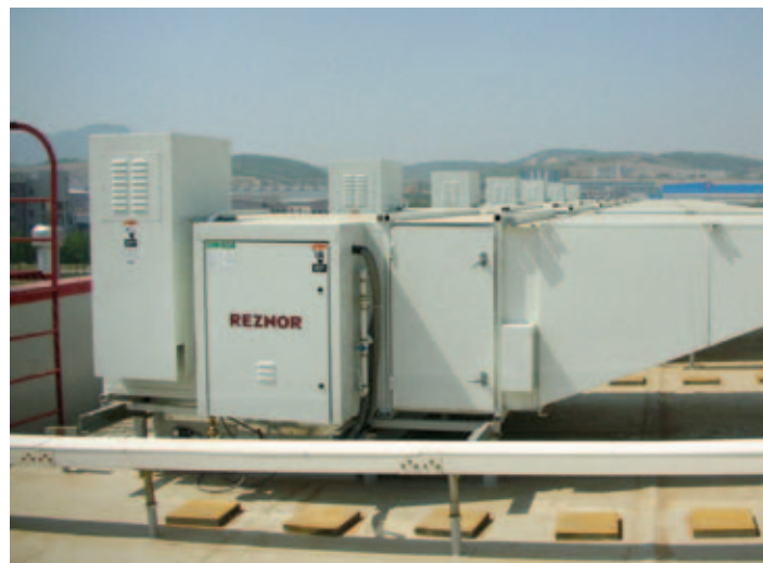
15 Reznor units grace the rooftop of Gibbs new manufacturing plant in Dalian, China.
